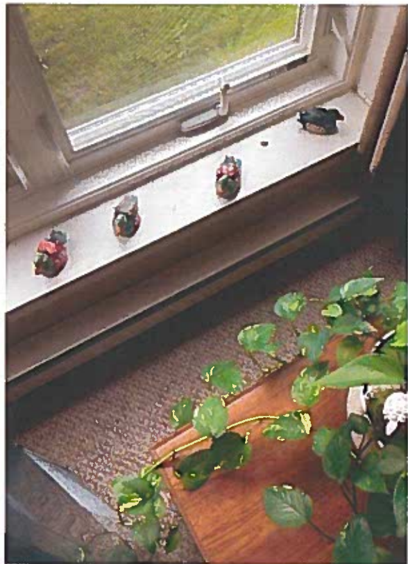
Figure 19: Typical in Suite Electric Baseboard Heater
