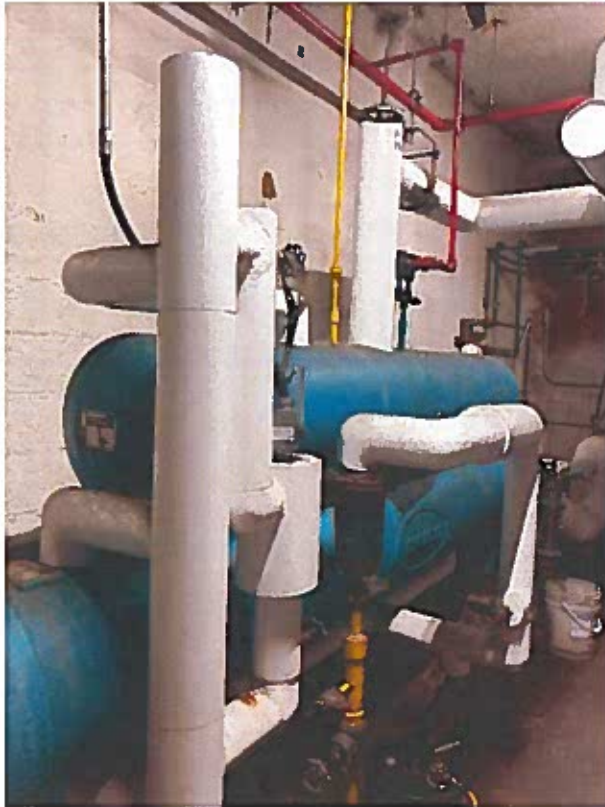
Figure 25: Ice Plant Compressors
