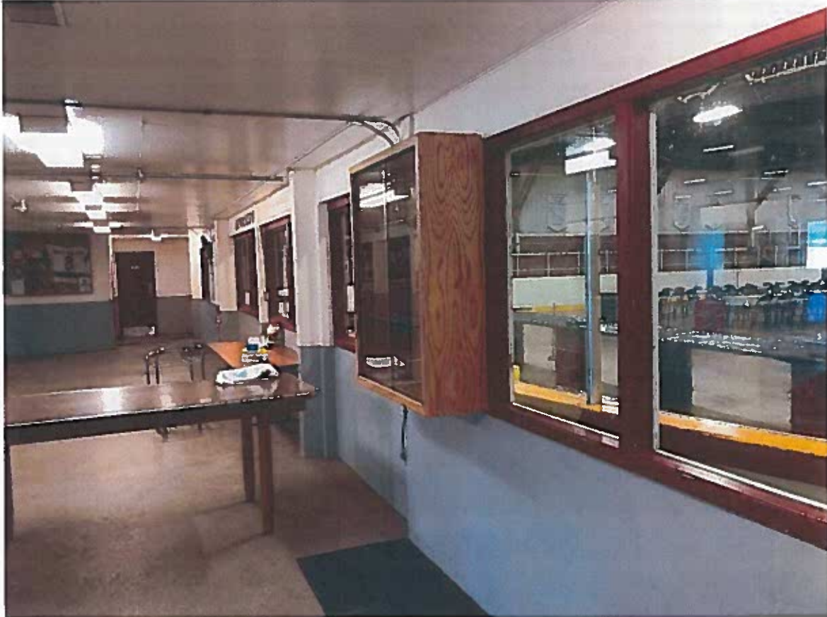
Figure 11: Common Area Single Pane Window to Unheated Arena
