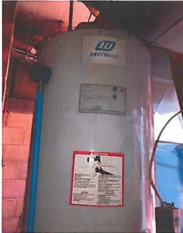
Figure 22: Domestic Hot Water Tank
