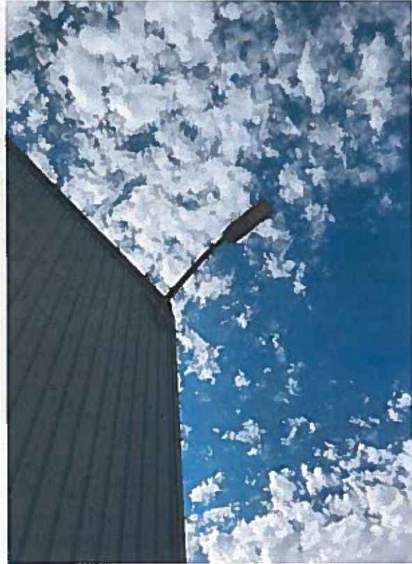
Figure 17: LED Parking Lot Lights
