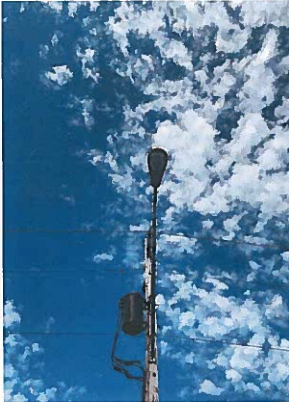
Figure 16: HPS Parking Lot Lights
