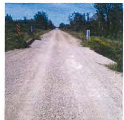
Crumbling single lane
