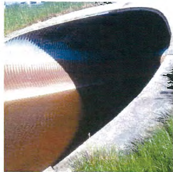
Large Diameter CSP Culvert
